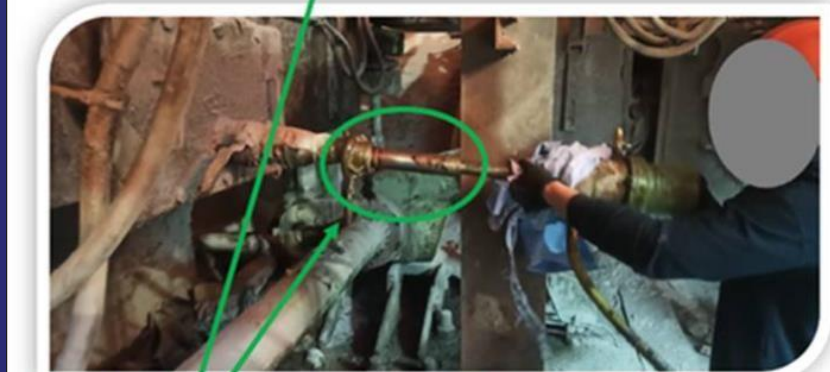
New designed mechanism for the coupling and operation of the pump in the sump
